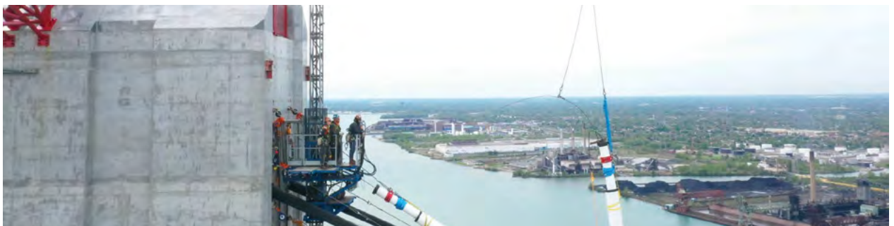
“View from the perch near the top of the Bridge” Photo courtesy of Dr. Murray Howe.
