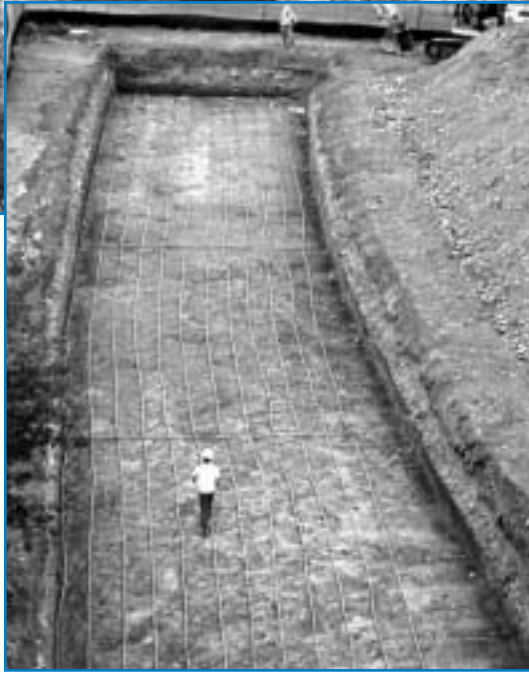
Workers install loop beds for GHES' phase 2 expansion. Geothermal systems absorb or expel heat in these loop beds.
